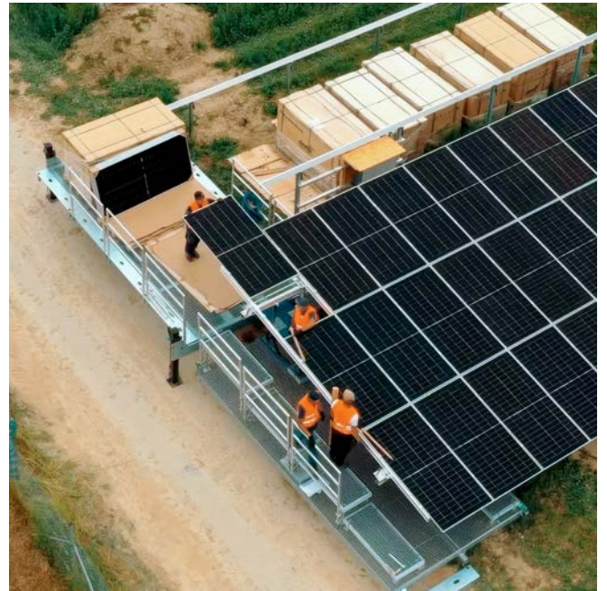
ASSEMBLY 2.0 in action: The solar modules are installed from the side – they are pushed on as a 'whole table' on rollers.
